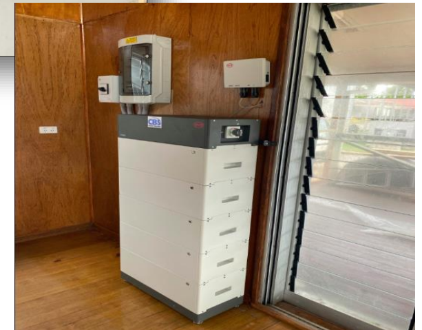
Demo Fale - 26kWp PV and 20kWh lithium-ion battery
