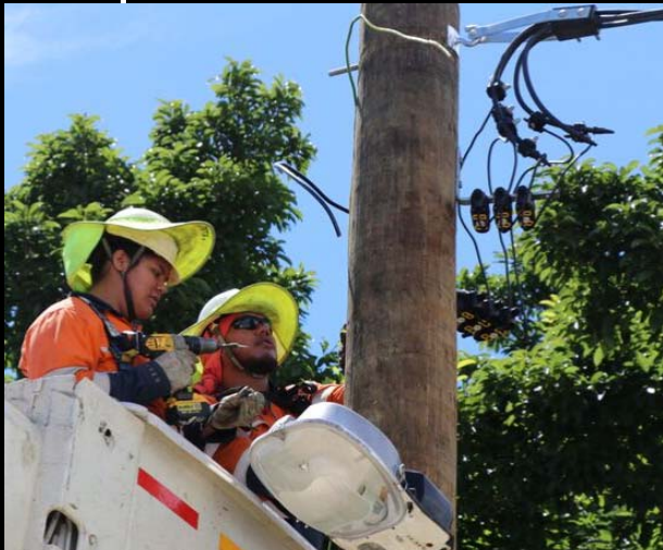
Increase network efficiency and reliability
